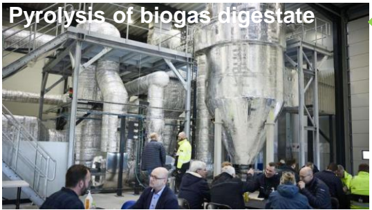
Pyrolysis of biogas digestate Stiesdal – SkyClean, Skive, Denmark (2023)
